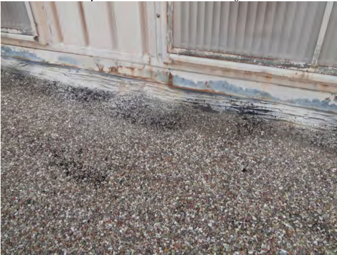
Photo #12 View of existing metal counter flashing at Bldg. B006 offset wall.
