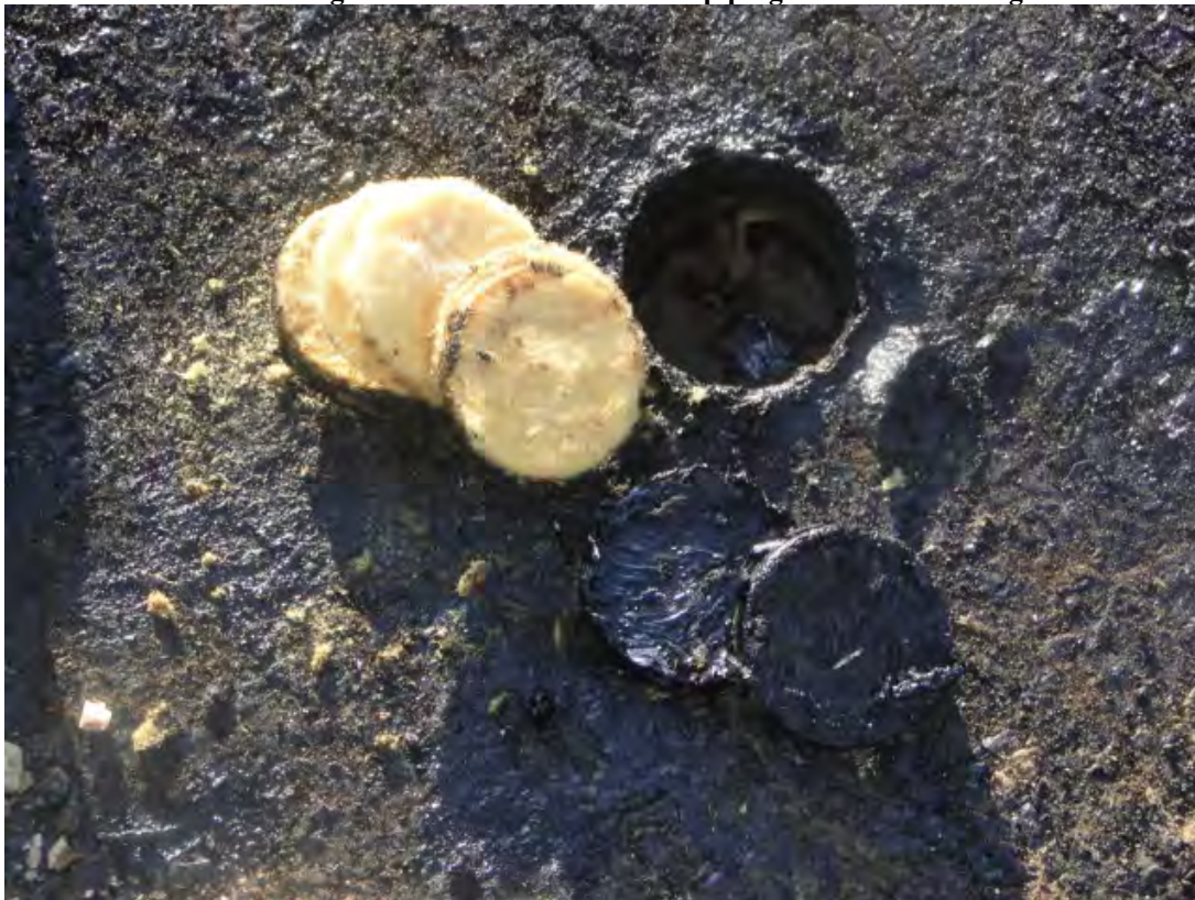
Photo #8 View of roof core cut at Bldg. B116. 1-1/2" Fiberglass insulation found on metal deck at perimeter roof.
