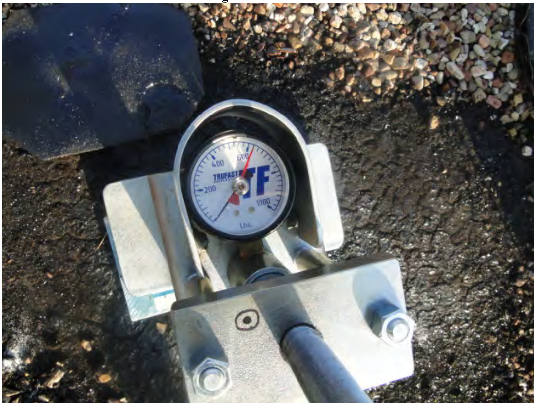
Photo #4 View of fastener pull test at Bldg. B006. Failure at 610 lbs force.
