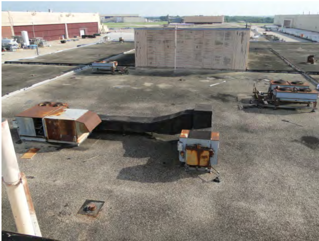
Photo #1 View of roof top mechanical equipment to be removed at Bldg. 116.
