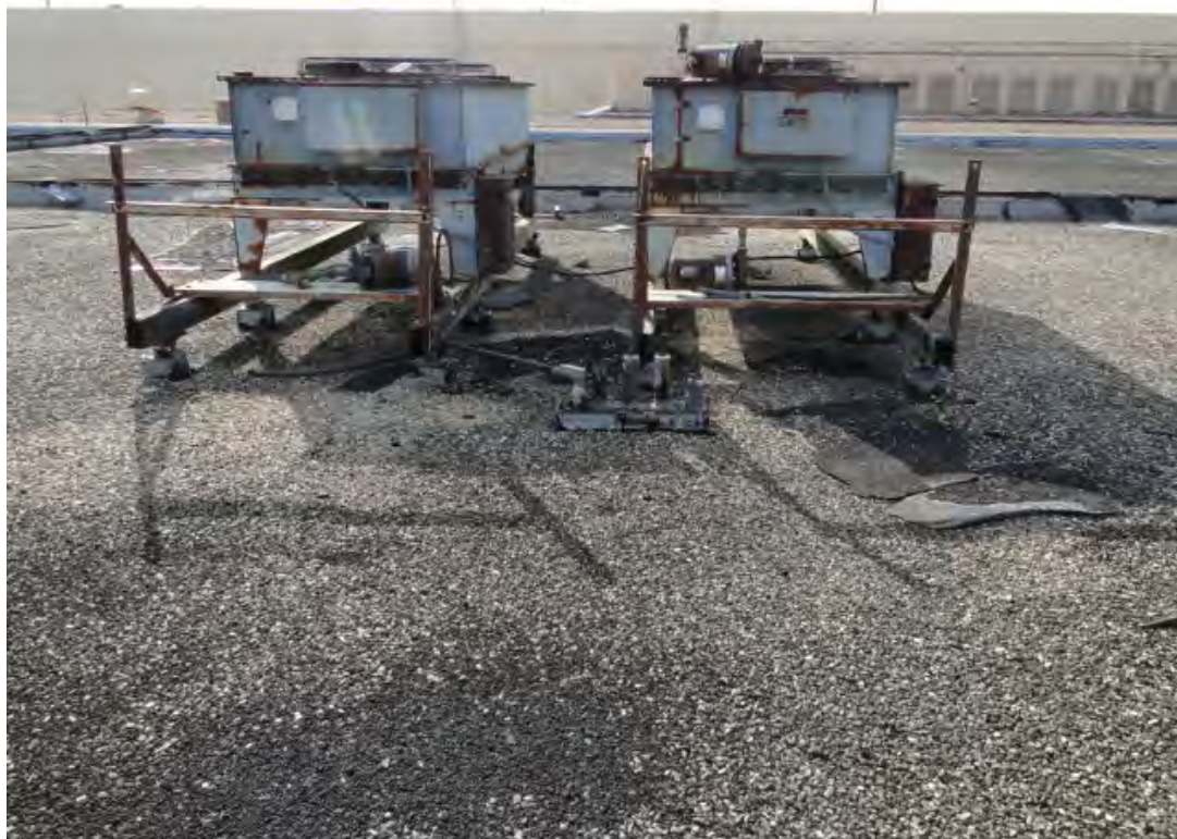
Photo #2 View of roof top mechanical equipment to be removed at Bldg. 116.
