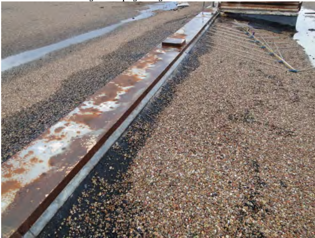
Photo #14 View of existing metal expansion joint between at Bldg. B005 & B006.
