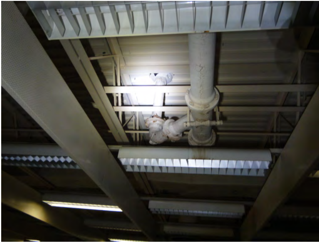
Photo #7 View of existing roof drain and storm sewer piping in the attic at Bldg. B116.
