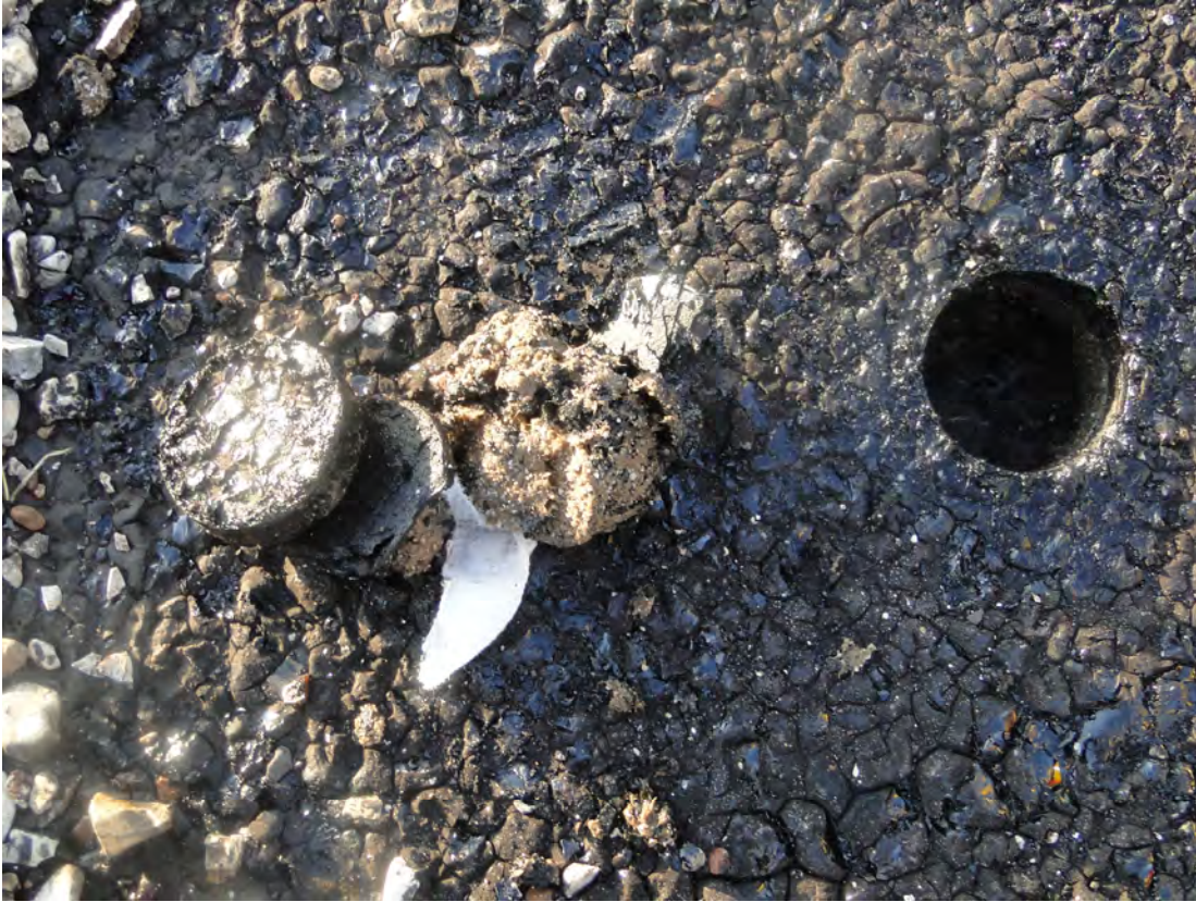
Photo #9 View of Perlite roof insulation at Bldg. B116 Roof Core Cut.
