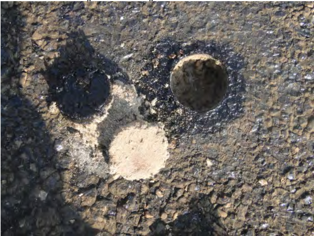
Photo #6 View of roof core cut at Bldg. B006. 1-1/2" Perlite insulation found on metal deck.
