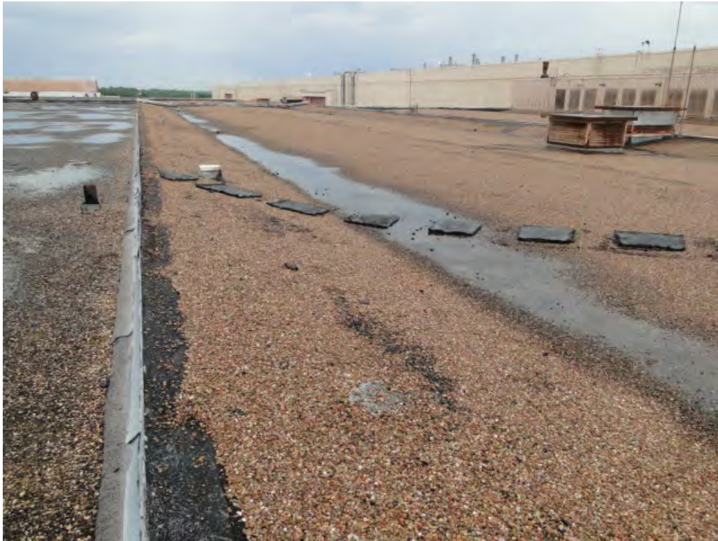
Photo #15 View of existing roof at expansion joint between Bldg. B005 & B006.
