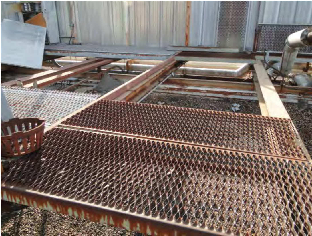
Photo #11 View of steel platform scheduled to be removed at Bldg. B005 & B006.
