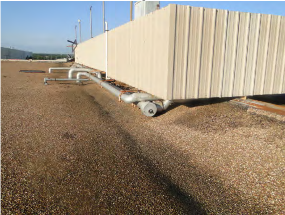
Photo #10 View of existing piping and metal siding to be removed at Bldg. B005 & B006.
